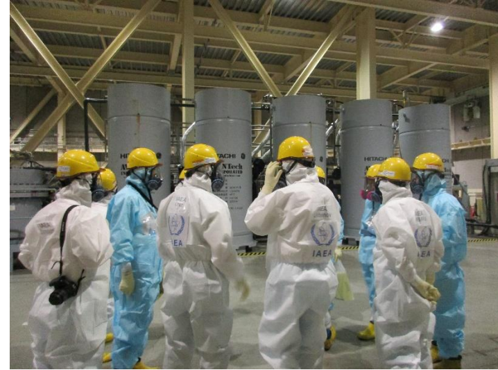
Water treatment facility for Subdrain
